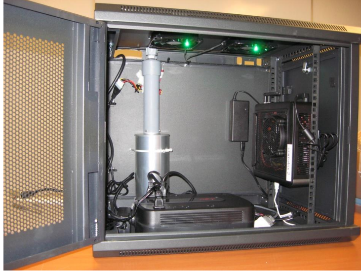
Figure 6) Housing for OPC, data logging system, modem, and UPS.
