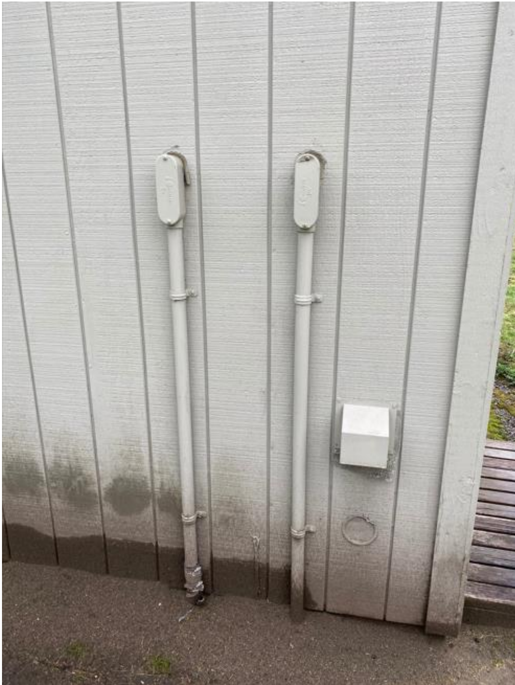
Electrical going into the building
