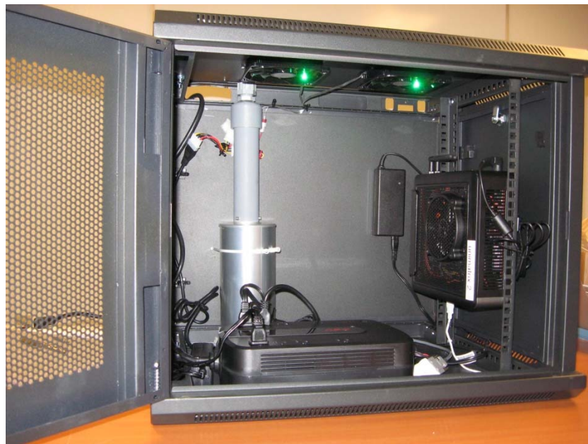
Figure 5) Housing for OPC, data logging system, modem, and UPS.
